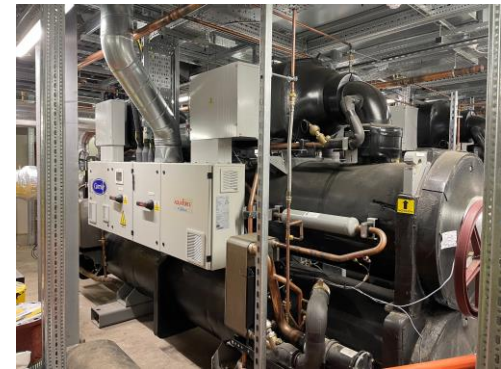
Figure 2.7: Citigen network energy centre plant – heat pump.
