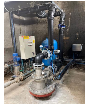
Figure 2.8: Citigen network energy centre plant above the ground source heat borehole.
